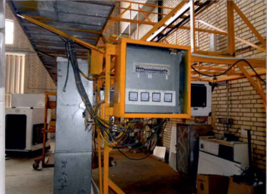
Control Panel For Testing Section
